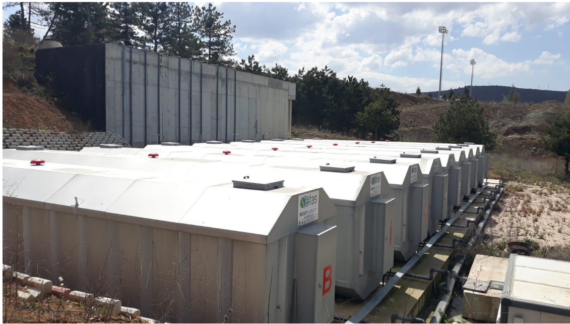
WWT Units, six packs total 900 m 3 /day
