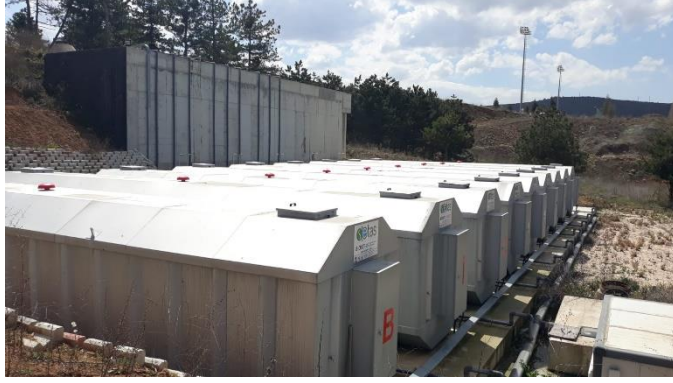
Biological Wastewater treatment plant with 900 m 3 /day capacity
